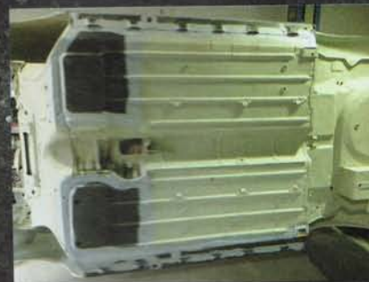
The front sections of the floors were replaced on both sides, along with the inner and outer sills.
